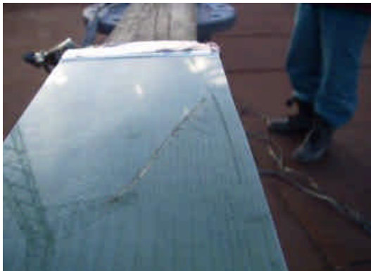
Fig.1 Lightning Damage in GFRP
